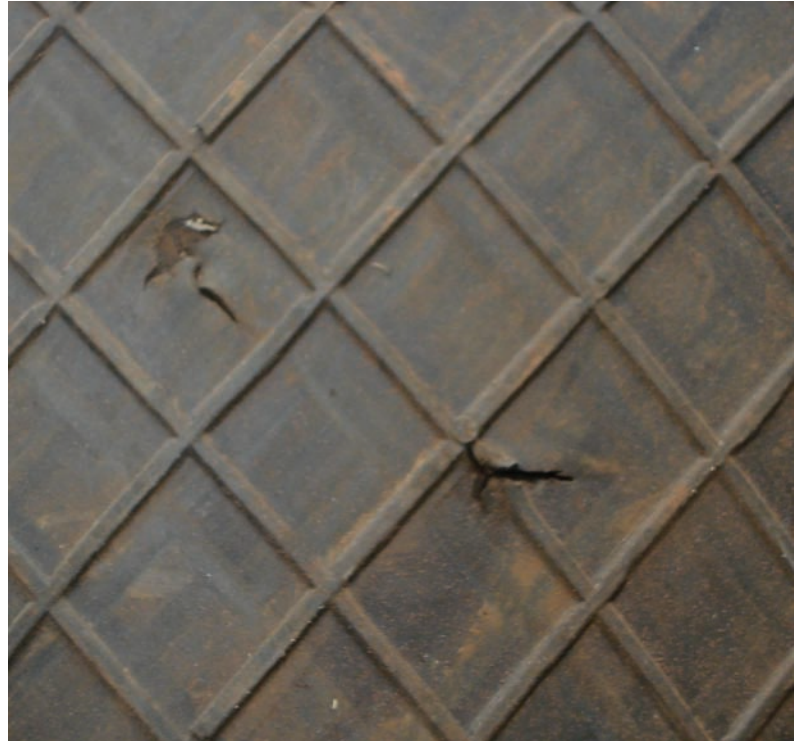
Tears in the cover caused by external, mechanical effects
